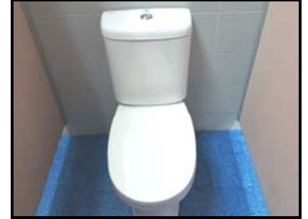
New water closet
